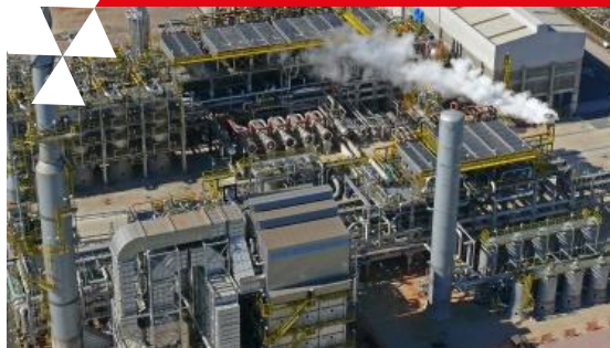
Mechanical Equipment 252,784 tons
